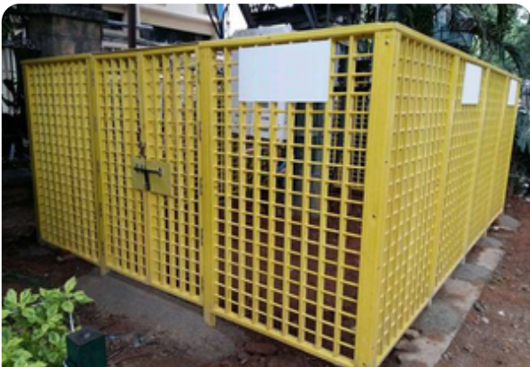
Electrical Substation Guardrail
